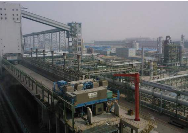
Shougang Jingtang Iron and Steel Plant – at which LanzaTech’s demonstration plant is situated; photo: wikimapia.org
